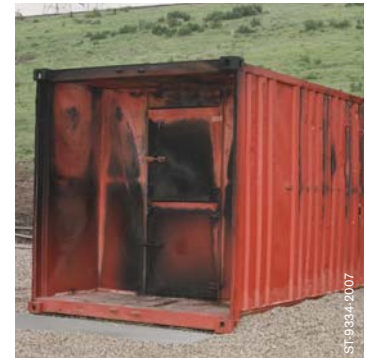
The Phase 3 System – Three year old unit in use at the Los Angeles Fire Academy.
